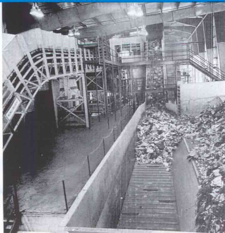
Rex apron conveyor delivers solid waste to shredder in this resource recovery plant.
